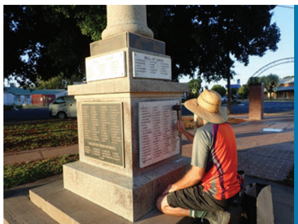
PHOTO: RGCRT Monumental-Heritage team member completing specialised traditional lead lettering work on the Bourke War Memorial, for Bourke Shire Council.
