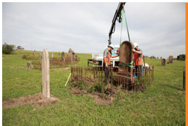
PHOTO: RGCRT Monumental-Heritage team members reinstalling the Edward Denny Day monument at Maitland Glebe Cemetery, as part of the conservation works program being undertaken by Maitland City Council at Glebe Cemetery. Police Magistrate Denny Day was notable for defying political pressures and successfully prosecuting a case against a gang of white colonists for the massacre of aboriginal women and children at Myall Creek. Photo Credit: 2018 Daniel Woo UXED.
